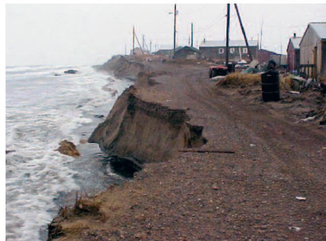
Fig. 15.18. Access road damage by coastal erosion, Shishmaref, Alaska (photo by Tony Weyionanna).
