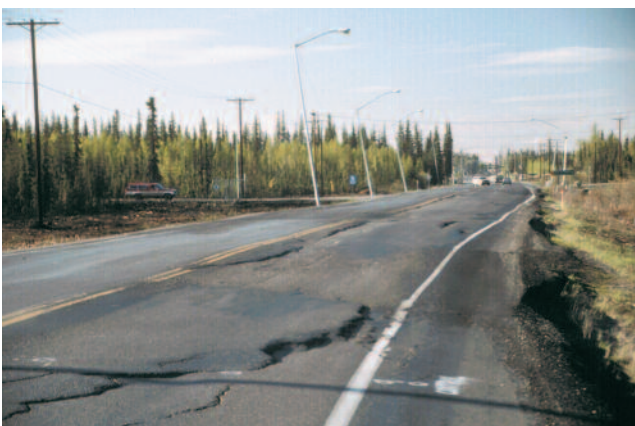
Fig. 16.20. Typical embankment cracking and differential thaw settlement in the discontinuous permafrost zone of Interior Alaska (Photo: Larry Hinzman, University of Alaska, Fairbanks).
