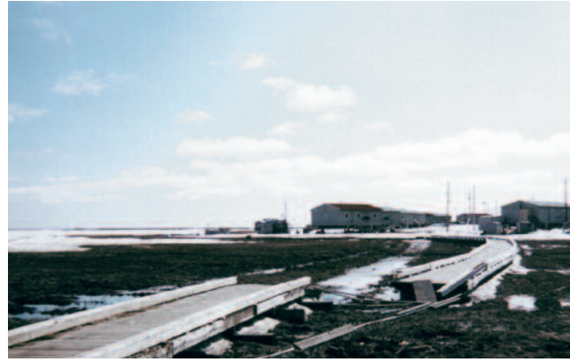
Fig. 15.14. Boardwalk damaged by storm surge flooding, Kipnuk, Alaska (photo by Mike Marcaurele).
