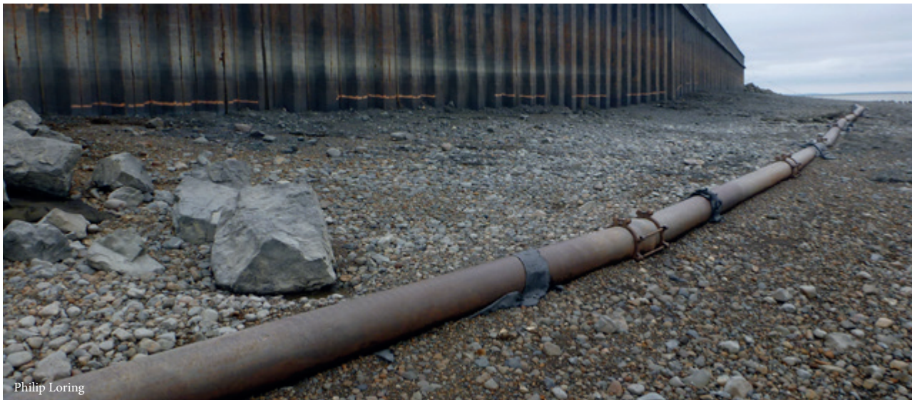
Philip Loring Seawall and sewage pipe exposed due to beach erosion in Dillingham, Alaska
