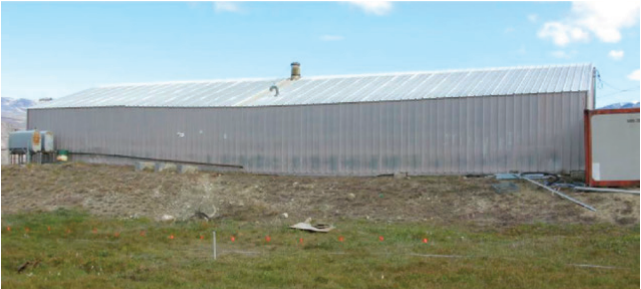
Figure 10.24 Municipal garage showing visible deformation (central depression) due to permafrost thaw settlement, Pangnirtung, Nunavut. Drillings next to this building revealed a very ice-rich surficial deposit (photo by E. L'Hérault).
